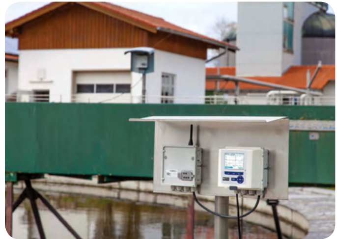
Optimal sludge level measurement with system 282/284 and wireless connection
